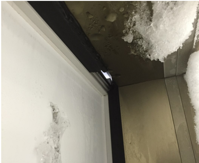
Damaged Gasket due to heater being turned off and door leaf freezing up
