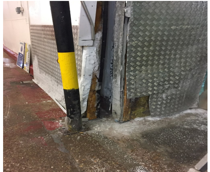
Sliding door damaged by impact
